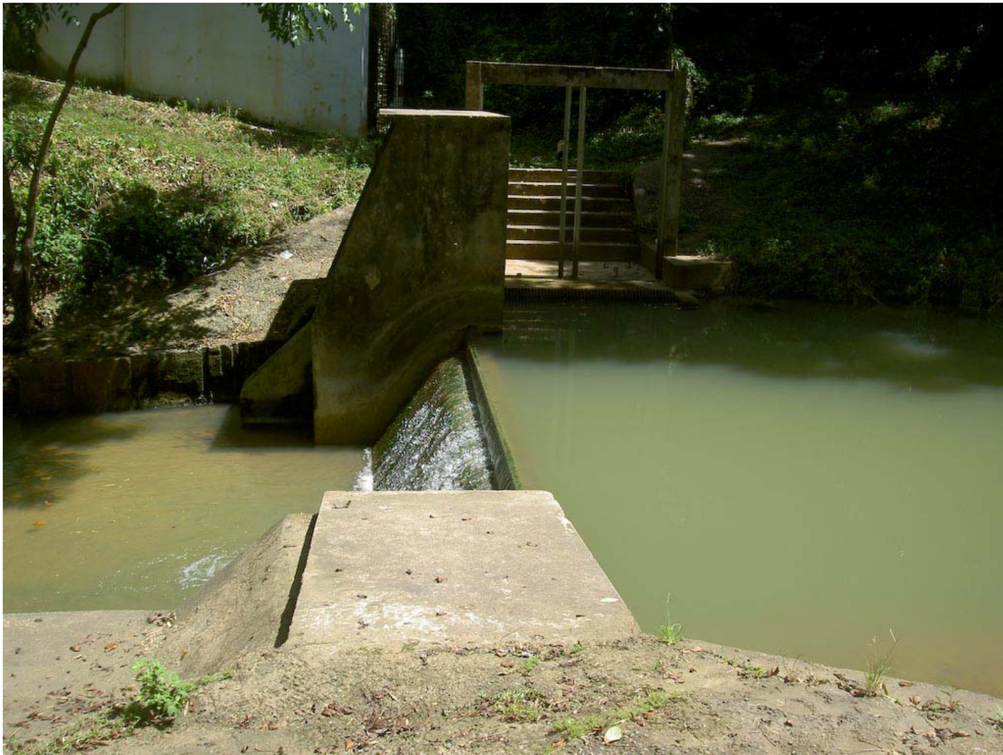
Río Guajataca pumped intake, Quebradillas
