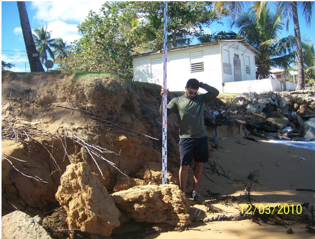
Figure 50. Severe erosion was measured in Playa Fortuna beach during December 2010 due by high swells.
